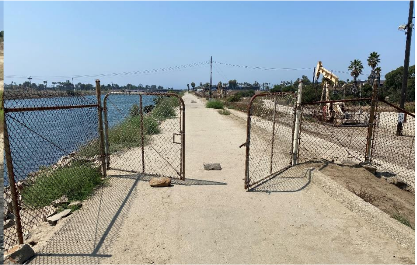
Levee gates left open
