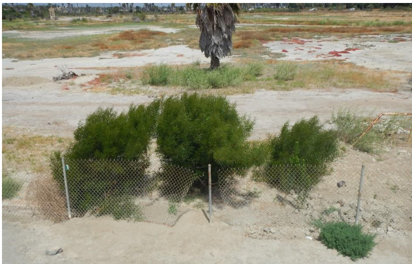
Fence line damaged in old encampment #1 location
