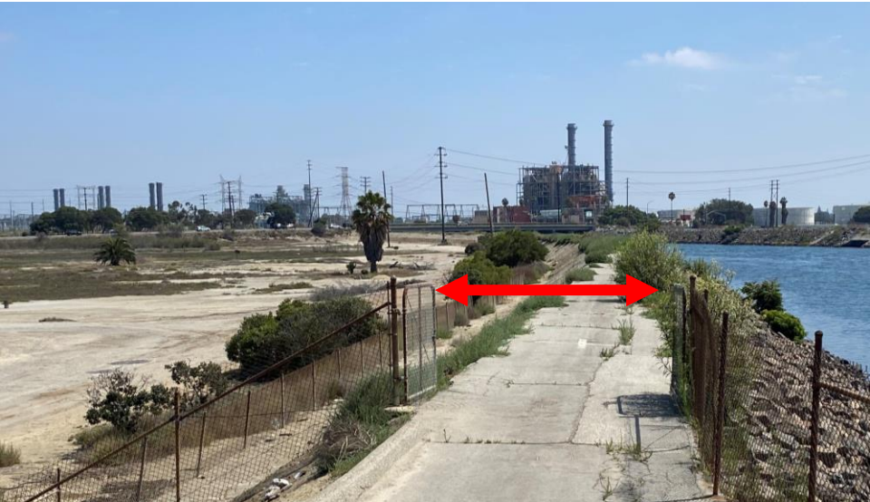
Levee gates left open
