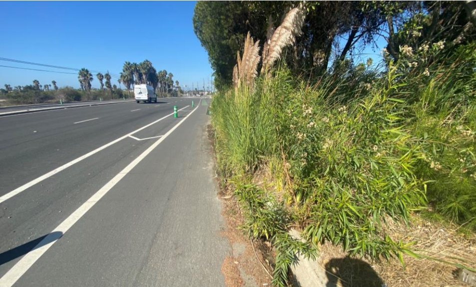
Vegetation encroaching bike path
