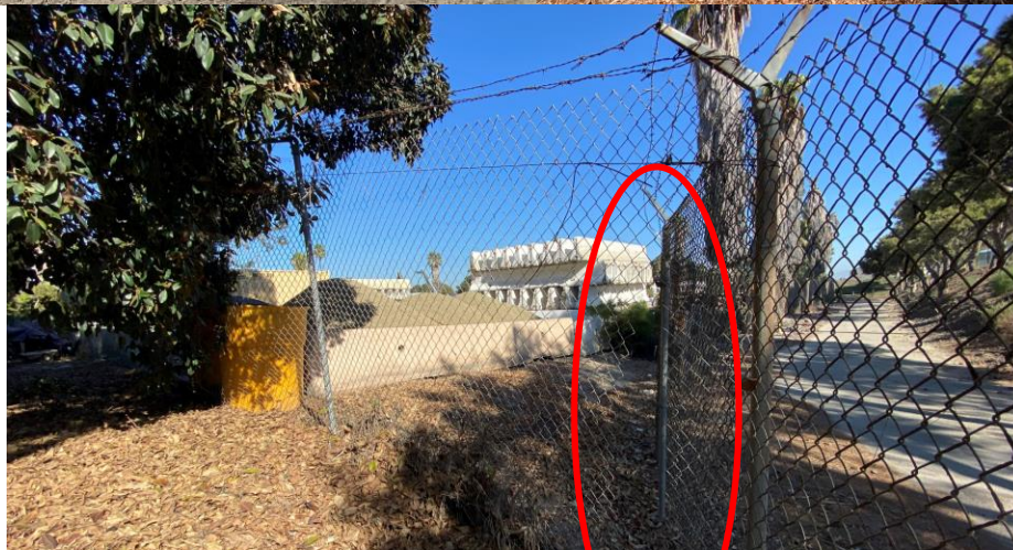
Fenceline breach in southeast corner of property
