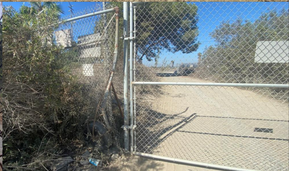
Fence line breach in northwest corner
