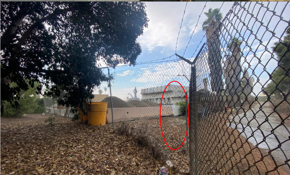
Fence line breach in southeast corner
