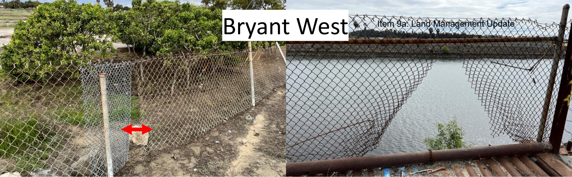
Breaches along southeast fence line
