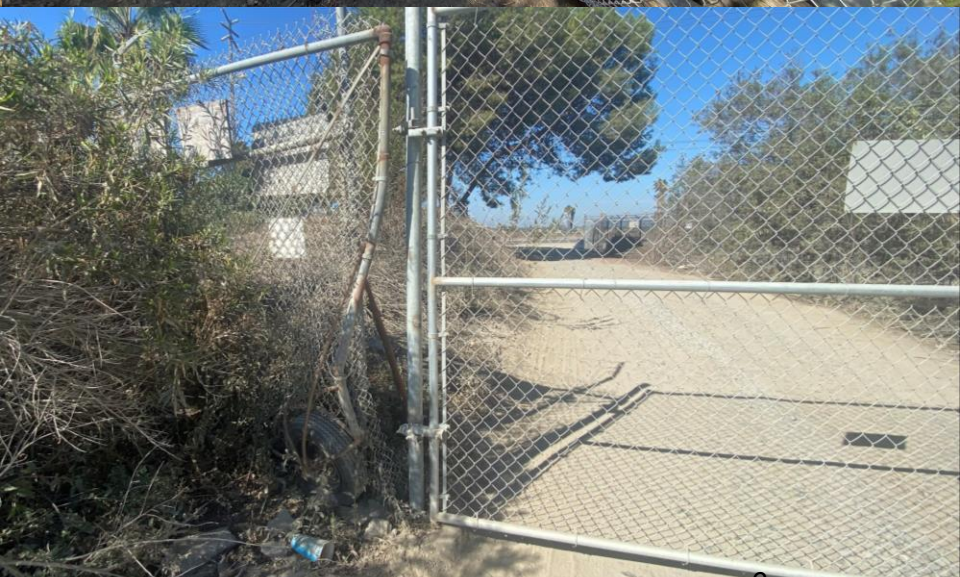
Fence line breach in northwest corner
