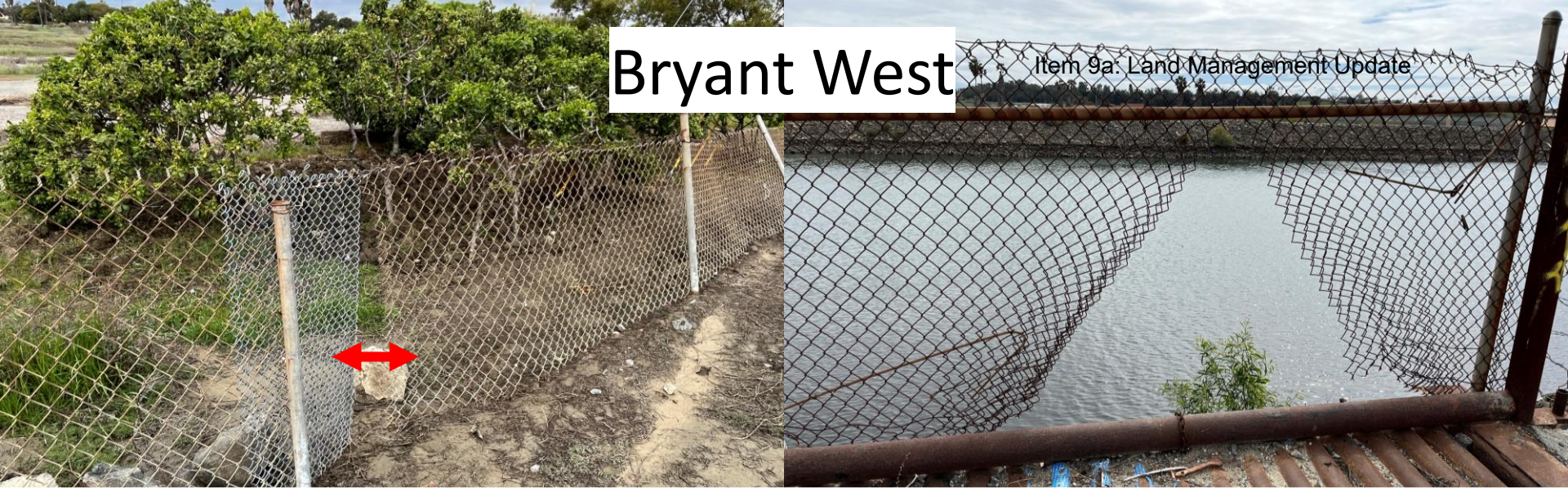
Breaches along southeast fence line
