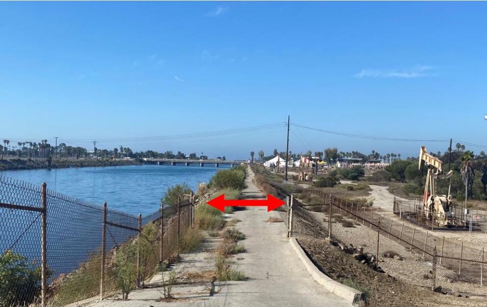
Levee gates found open
