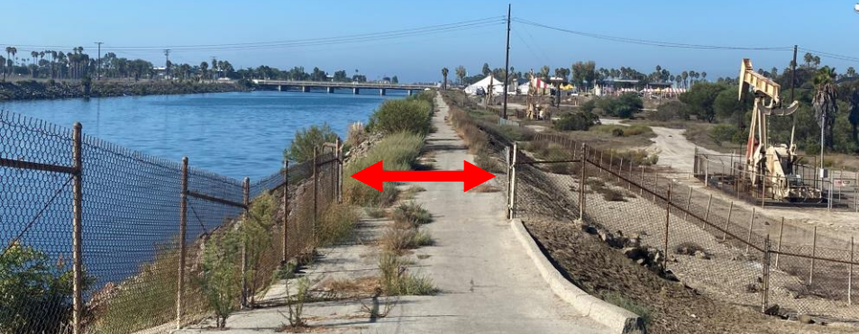
Levee gates found open
