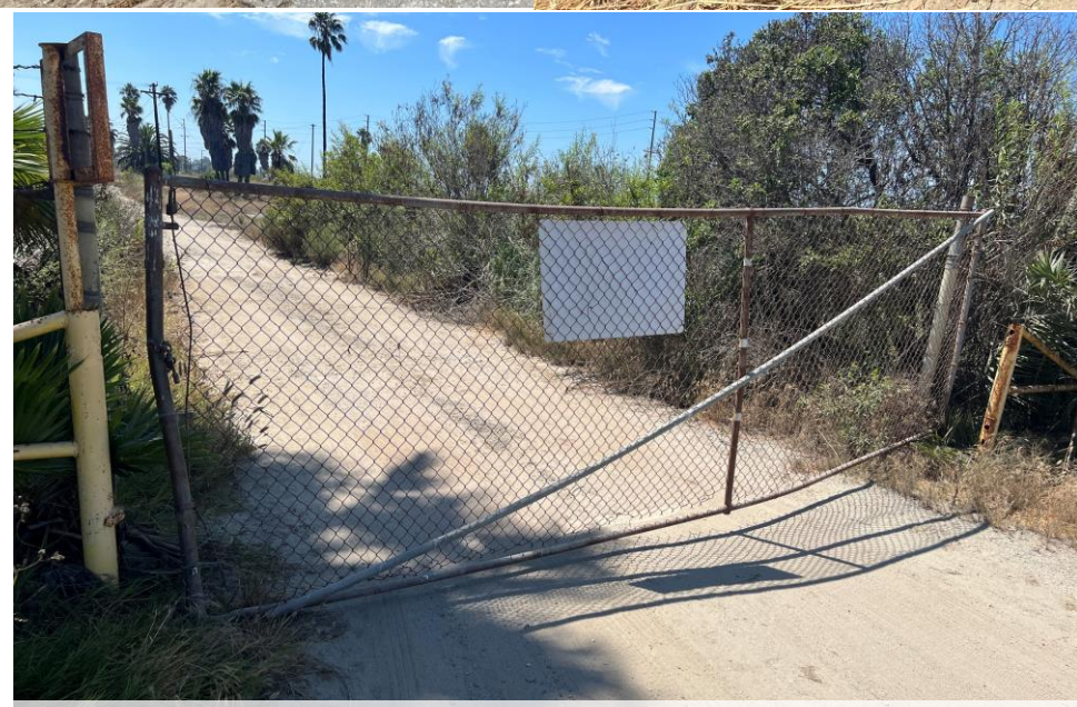
Entrance gate damaged
