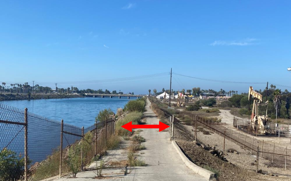
Levee gates found open
