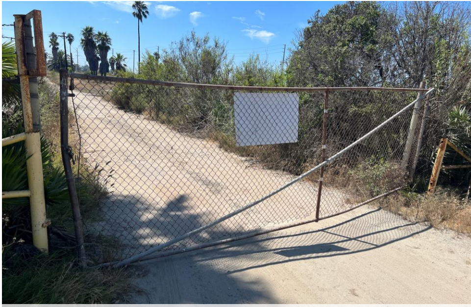
Entrance gate damaged
