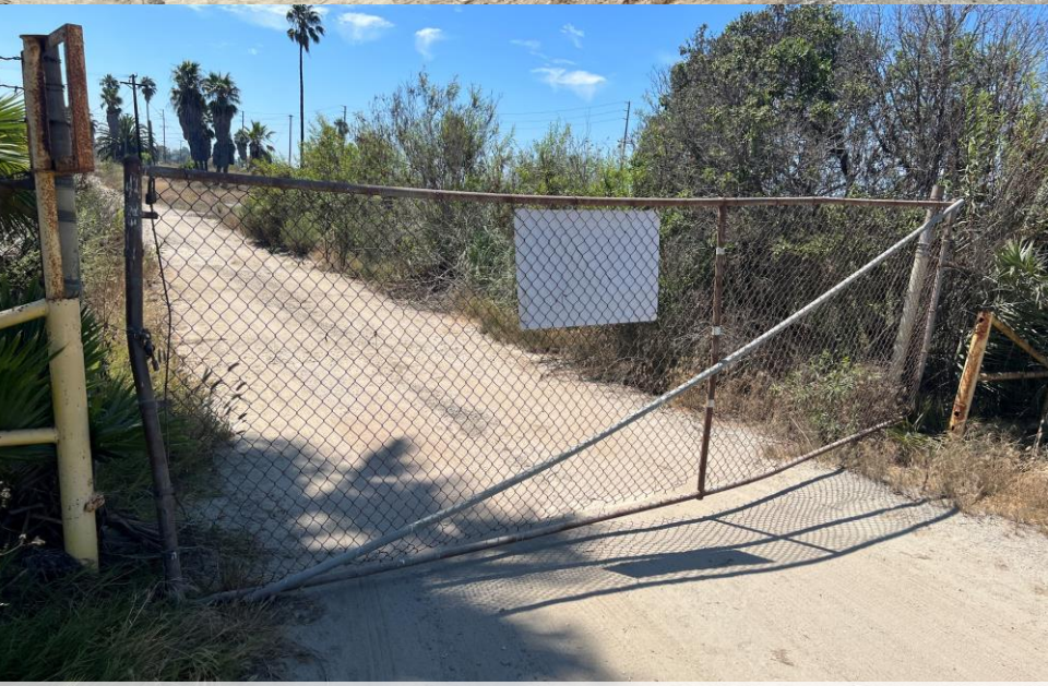
Entrance gate damaged
