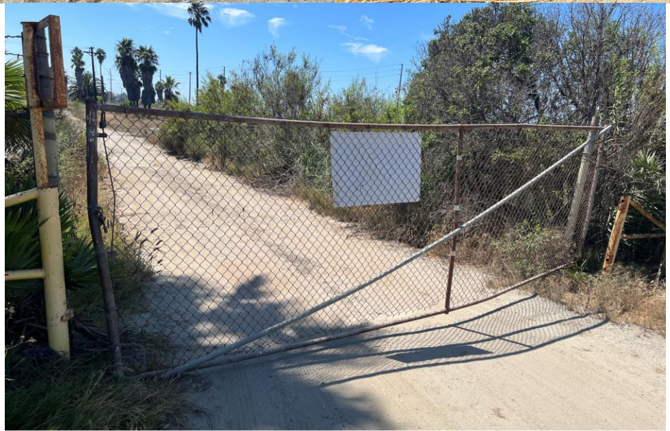
Entrance gate damaged
