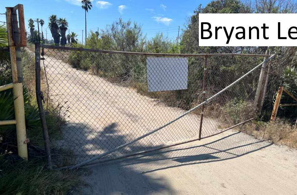
Entrance gate damaged
