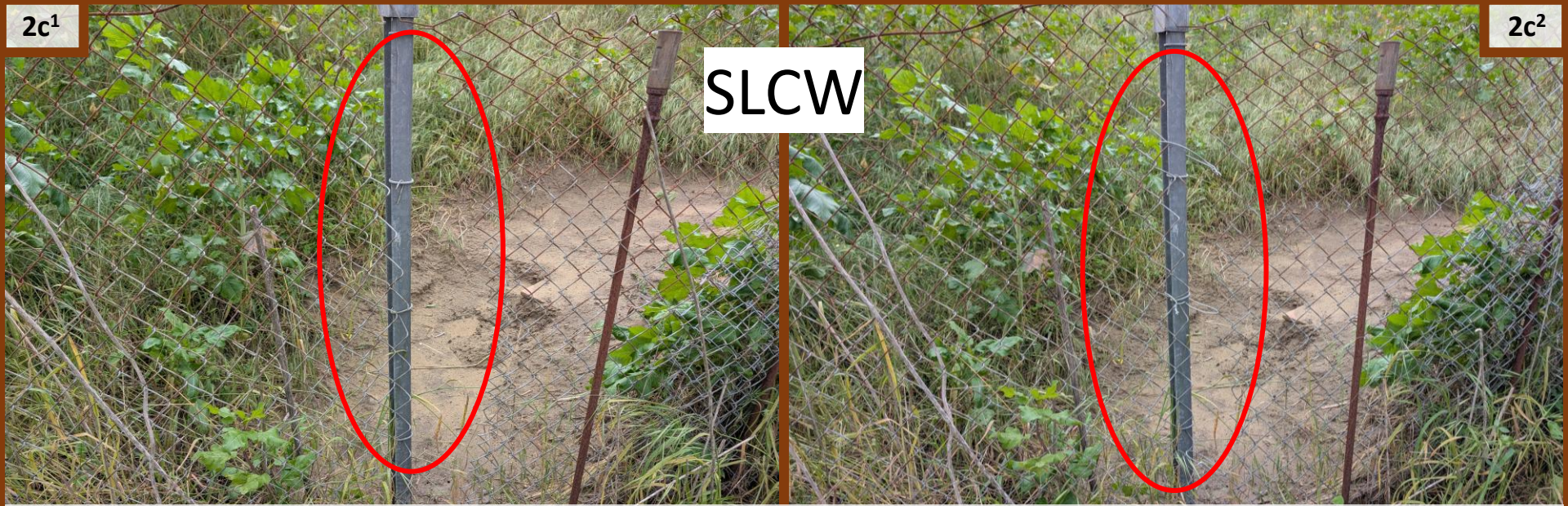
Patched hole in fence separating property from Gum Grove Park parking lot.
