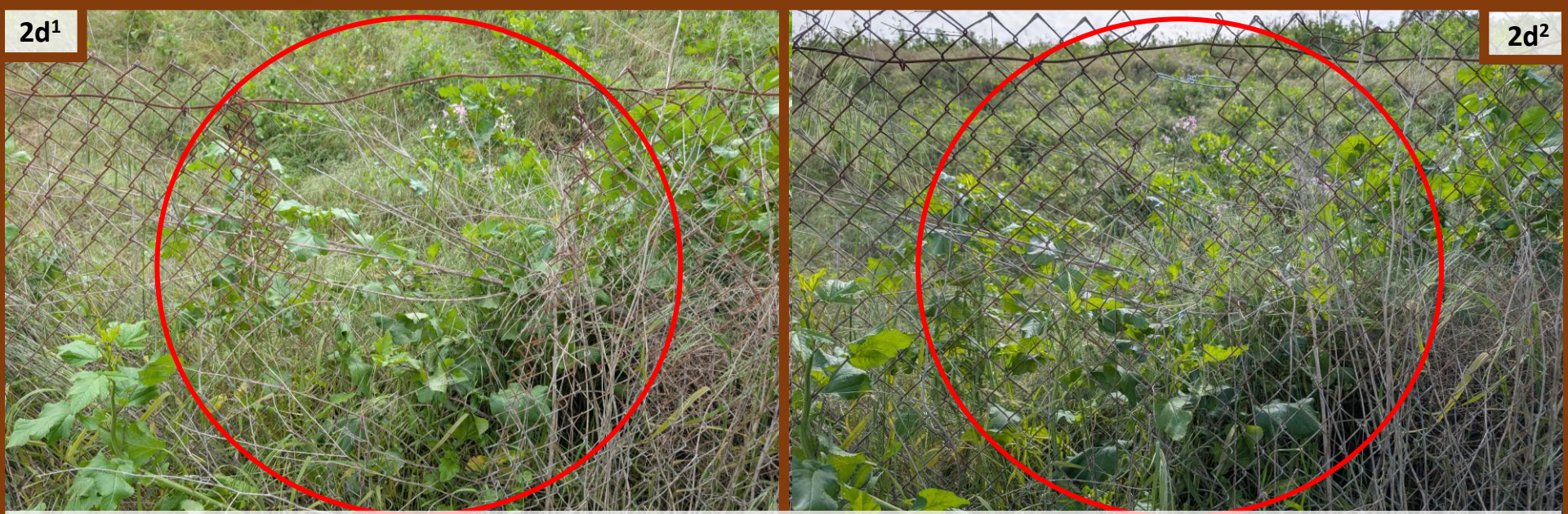
Patched hole in fence separating property from Gum Grove Park.
