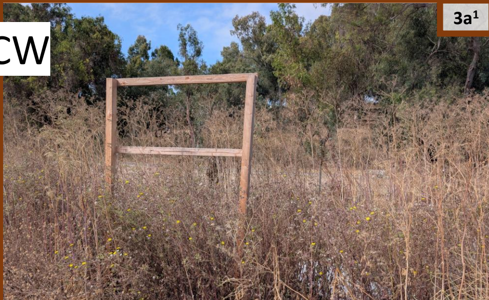
LCWA sign facing Gum Grove Park has fallen over.
