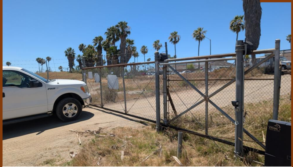
Faulty motion sensor preventing gate from opening.
